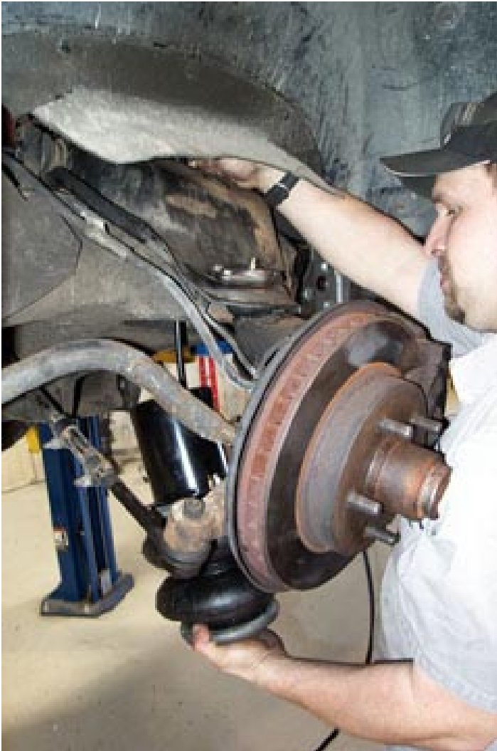
The air line is installed in the spring fitting before sliding the spring in place because you can't get to it afterward.
